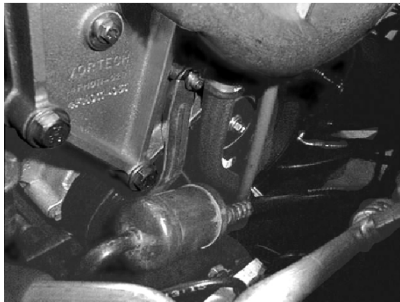
Fig. 8.2-g / Air Conditioning Silencer
